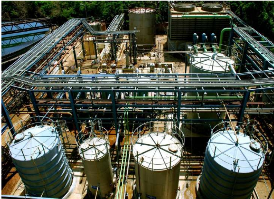
PRETREATMENT AREA OF CHLOR ALKALI PLANT
