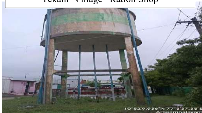
Arasampalayam Village –Water tank
