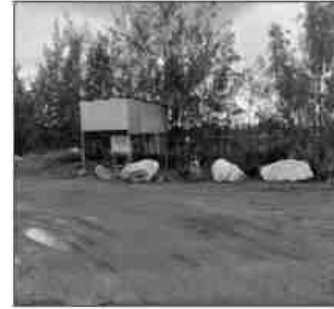
S3 – Power panel shed – Within M.L
